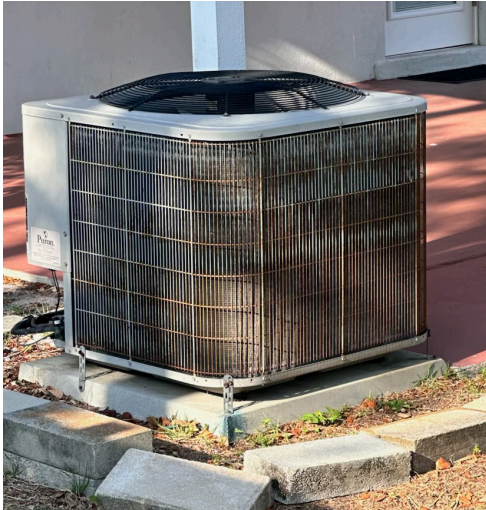
Unit left unprotected. Installed Spring 2021.
