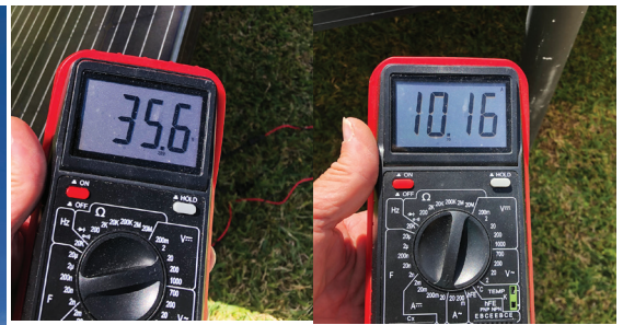
After cleaning: 35.6V x 10.16A = 362W
