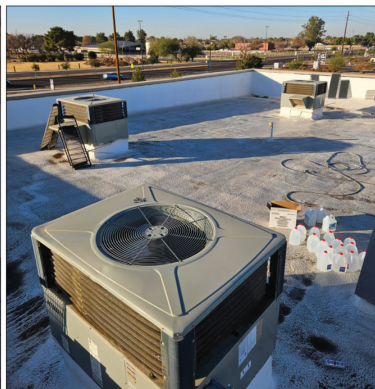
Three of ALA Gilbert's Trane 4-ton units
