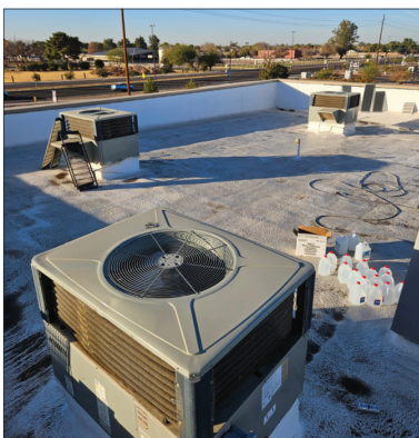
Three of ALA Gilbert's Trane 4-ton units
