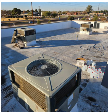
Three of ALA Gilbert's Trane 4-ton units
